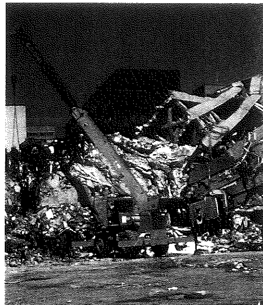
FIGURE 12 Destructive Power of Resonance In the 1985 earthquake in Mexico City, resonance caused the greatest damage to buildings between 8 and 18 stories tall. Inferring Why did taller buildings survive the earthquake?
